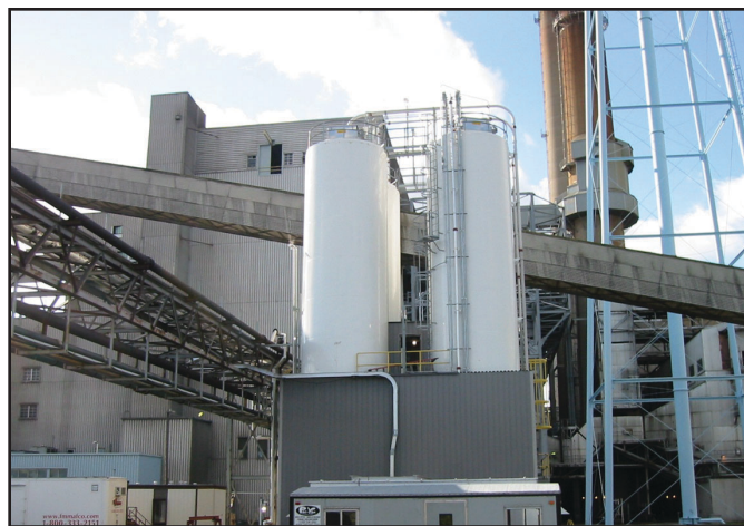
Figure 6: Consumer's Energy Plant Karn
