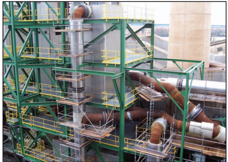
Figure 1: The pulse-jet baghouse and SCR de-NO x tower portion of the Mercury Research Center located at Gulf Power Company's Plant Crist Unit 5.
