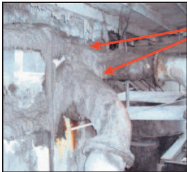
Figure 1: Solids Build up on Tank and Top of Piping
