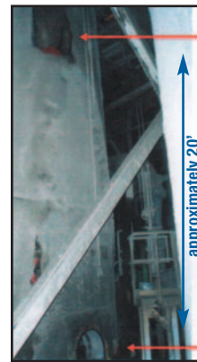
Figure 2: (Top arrow) Dried Slurry Fell from Tank. (Bottom arrow) Manhole Entry
