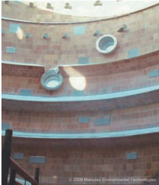
Figure 1: Absorber Liquid Redistribution Devices (ALRD) in tile-lined FGD
