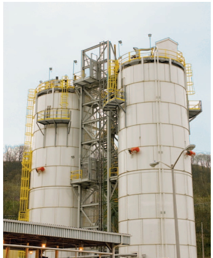
Figure 20: PAC Injection Silo [3] .
