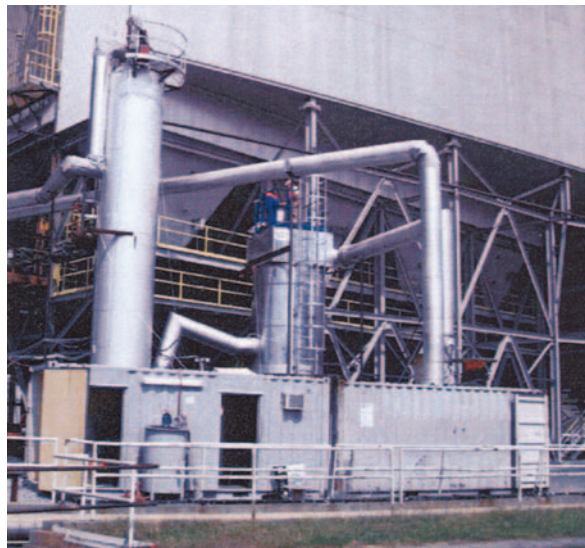
Figure 17: IAQCS Pilot Plant
