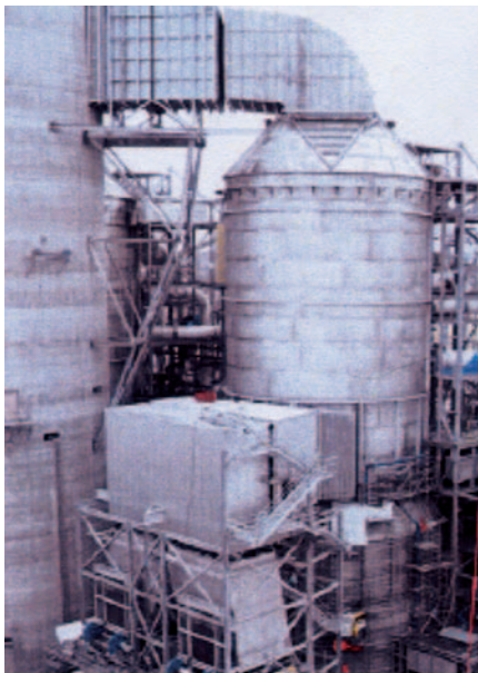
Figure 12: Spray Tower Absorber
