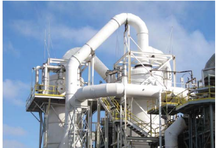
Figure 12: Two-Stage Membrane WESP Modules at Climax Acid Plant
