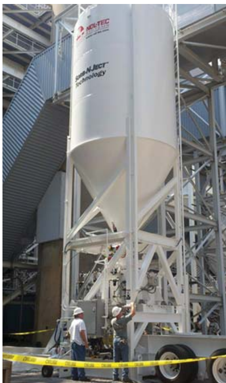
Figure 26: In field tests, DSI is proving its ability to meet new EPA standards.
