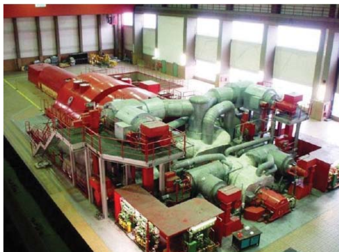
Figure 9 – Turbine Deck at Ibbenbüren Plant
