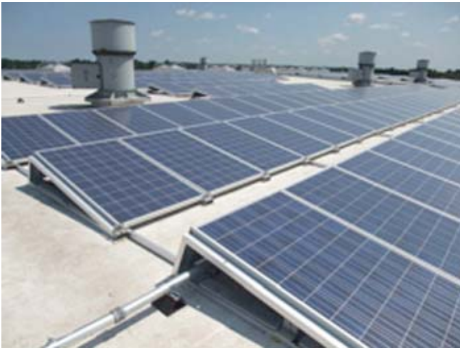
FIGURE 5: Roof-top PV array (Montgomery County, MD)
