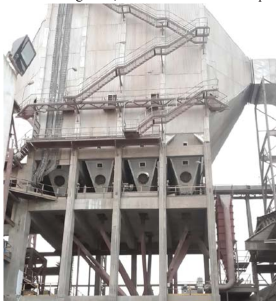
FIGURE 16: MHIPL Sree Jayajothi Cements Limited clinker cooler ESP with 4 fields - side view
