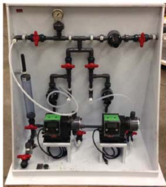
FIGURE 38: Photo of Simple Coal Additive Skid
