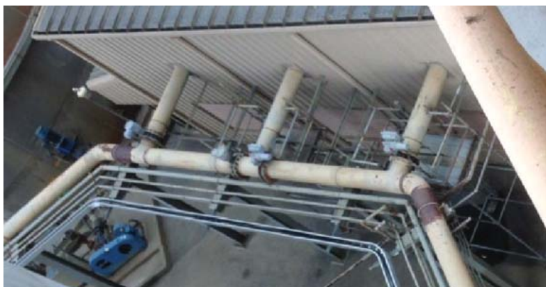
FIGURE 43. Forced Oxidation Air Configuration with Blowers Dedicated to Two Absorbers and a Common Spare
