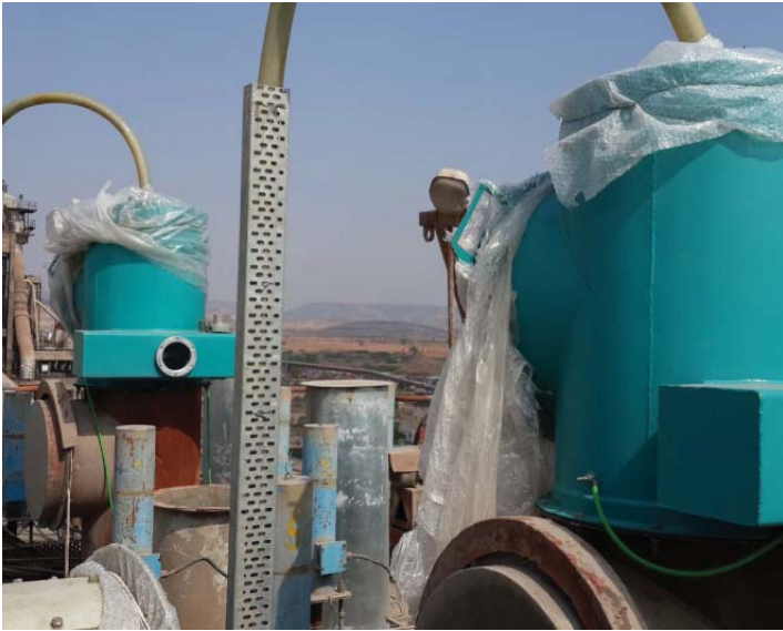
FIGURE 18: ModuPower™ MPX Ground switches mounted on ESP roof. HV cable penetration from top
