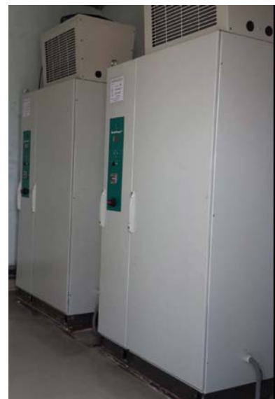
FIGURE 17: 2 x 60 kW ModuPower™ MPX cabinets mounted remotely in control room. 100kV rated HV cable used to connect MPX to ESP.
