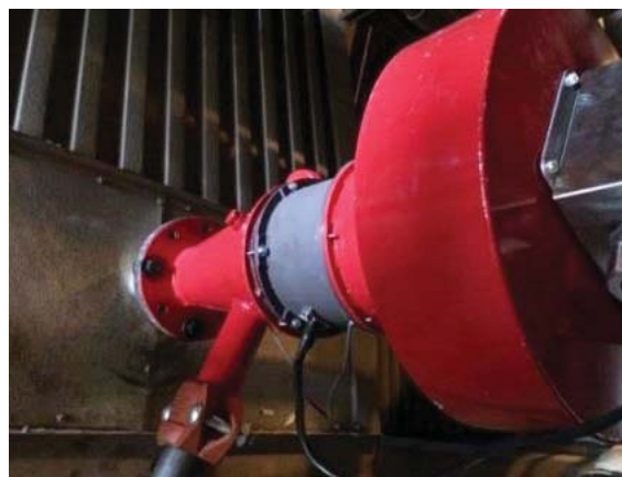
Figure 18: Image of Sorb-Tec Lanceless Injection Technology installed on a major utility-scale coal-fired power plant.
