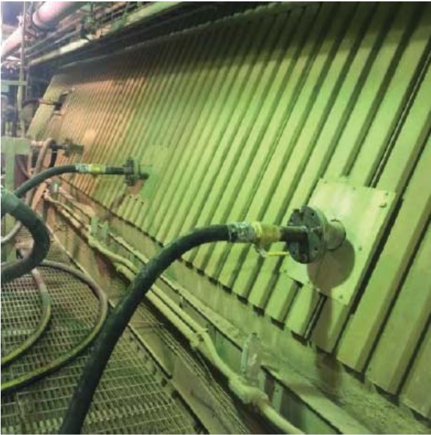
Figure 32: Lances installed on the B side duct
