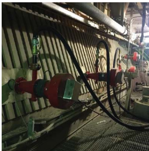
Figure 31: Sorb-Tec installed on the A side of the duct
