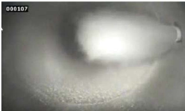
Fig 20: Image taken by an in-duct camera demonstrating the effect of Sorb-Tec on a major utility-scale coal-fired power plant.
