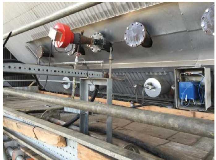
FIGURE 29: One (1) Sorb-Tec injector installed on the A side of the duct.
