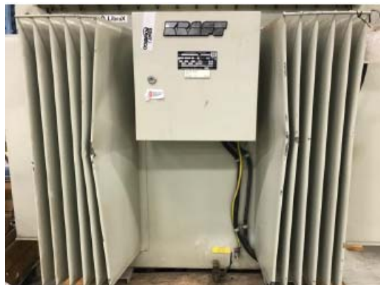
Figure 26: Physical damage to T/R cooling fins
