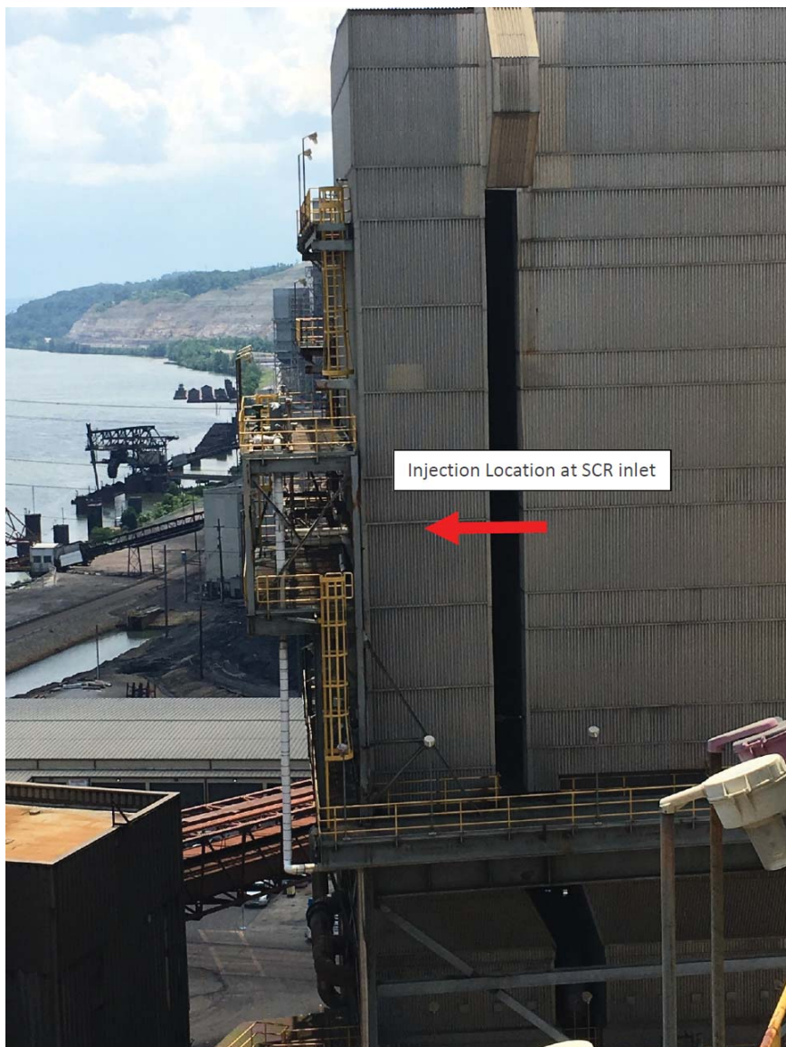
Figure 26: Elevation view of SCR inlet duct. Injection occurred at the location noted above.
