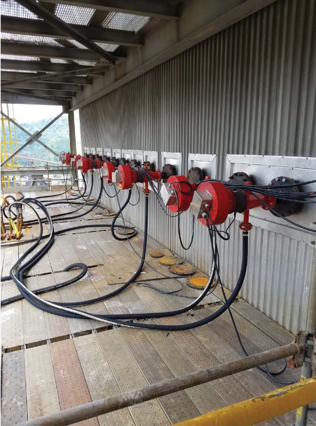
Figure 25: Test set up at SCR inlet. Eight (8) Sorb-Tec units were installed to maximize dispersion of the sorbent.
