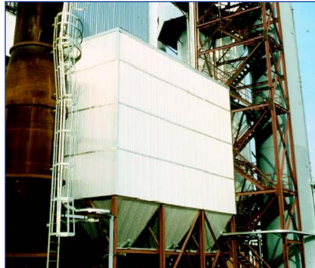
Coal-fired Industrial Boiler 110,000 ACFM
