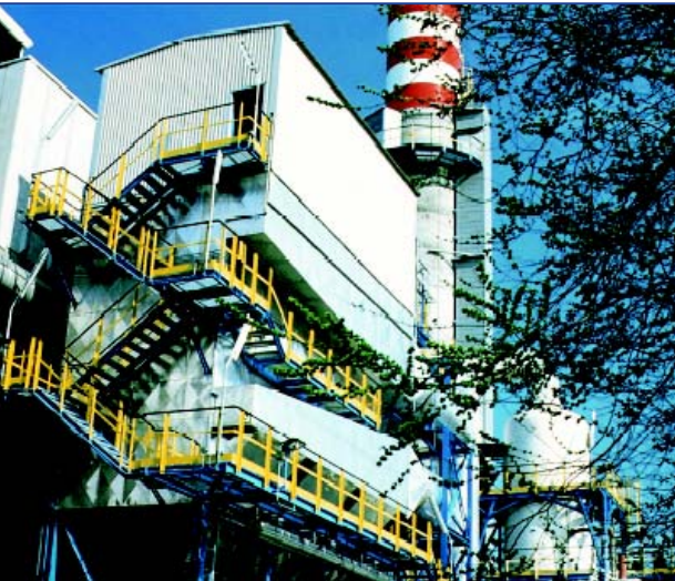
Municipal Solid Waste Incineration 16 MW – 65,000 ACFM
