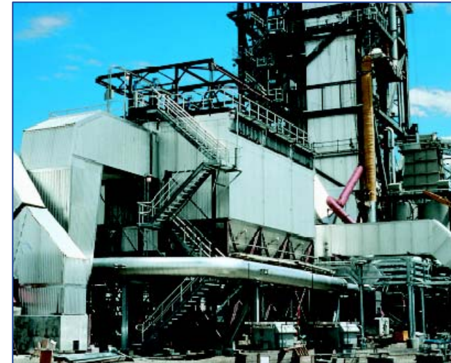
Utility Boiler 500,000+ ACFM
