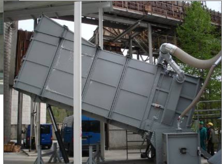
Container placed within fully enclosed vented enclosure
