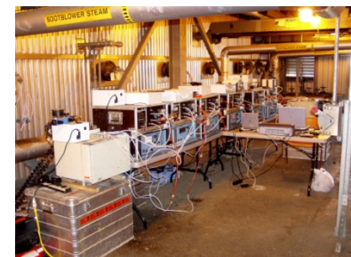
Multi-point NO x /O 2 Analyzer Set-up
