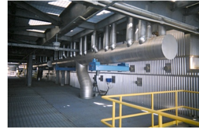
Ammonia Header And Take-Off Trunks
