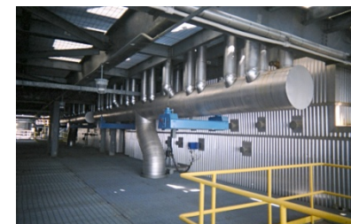
Ammonia Header And Take-Off Trunks
