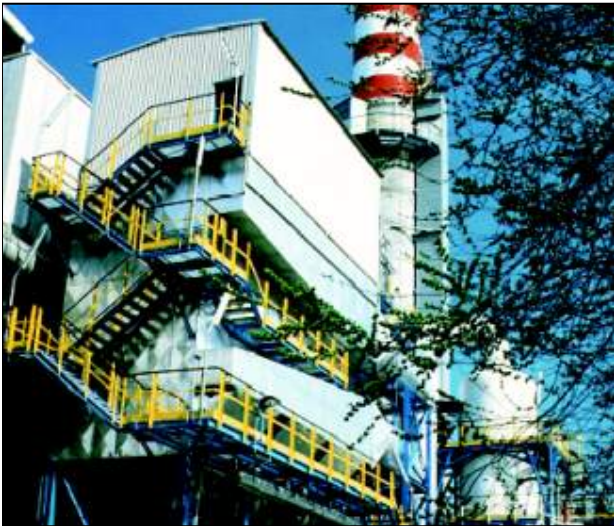
Municipal Solid Waste Incineration 16 MW – 65,000 ACFM
