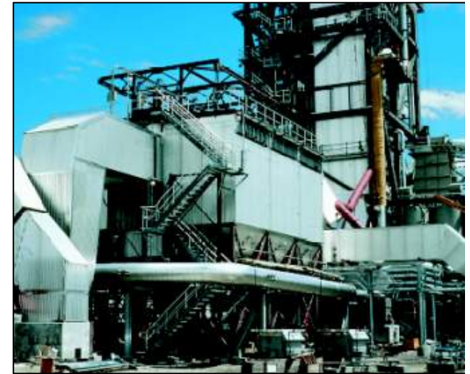
Utility Boiler 500,000+ ACFM
