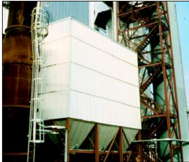
Coal-fired Industrial Boiler 110,000 ACFM
