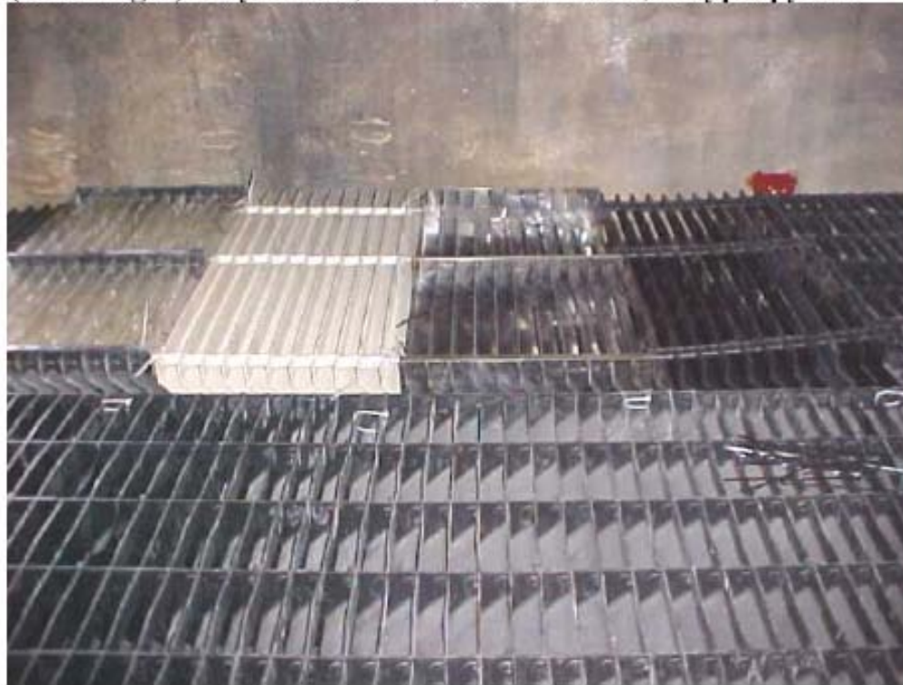
Figure 2. Test Installation at APS's Cholla Station, Unit 2: Materials (left to right) Polysulfone, FRP, Stainless Steel, Polypropylene
