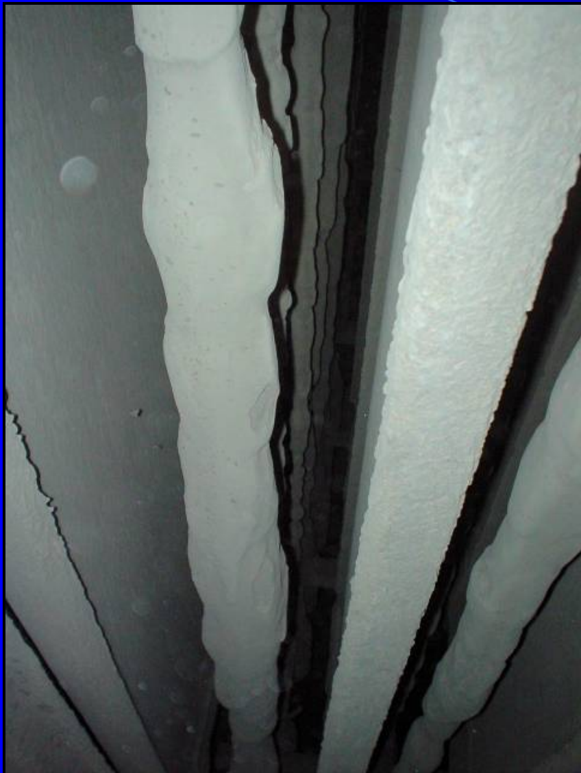
Excessive Emitter & Plate Ash Buildup
