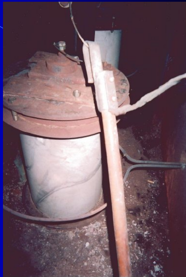
Cracked Support insulator
