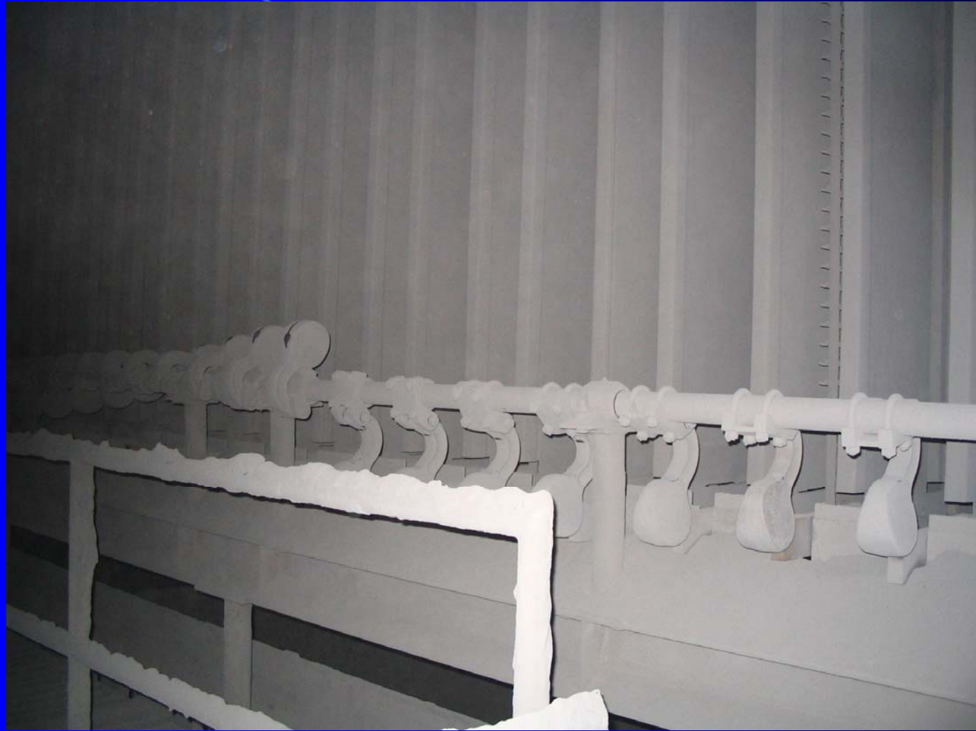
Rotating Hammer Rapping System
