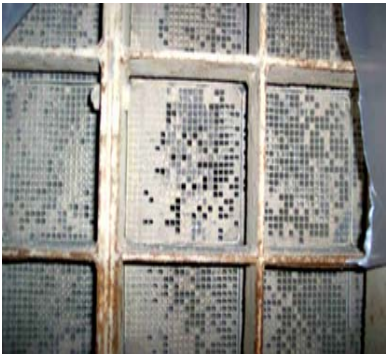
LPA Plugged Catalyst – STEAG's Voerde Power Station
