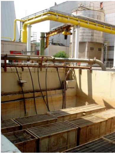
Rejuvenation Tank at Weiher Power Station
