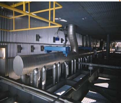
Ammonia Header And Take-Off Trunks
