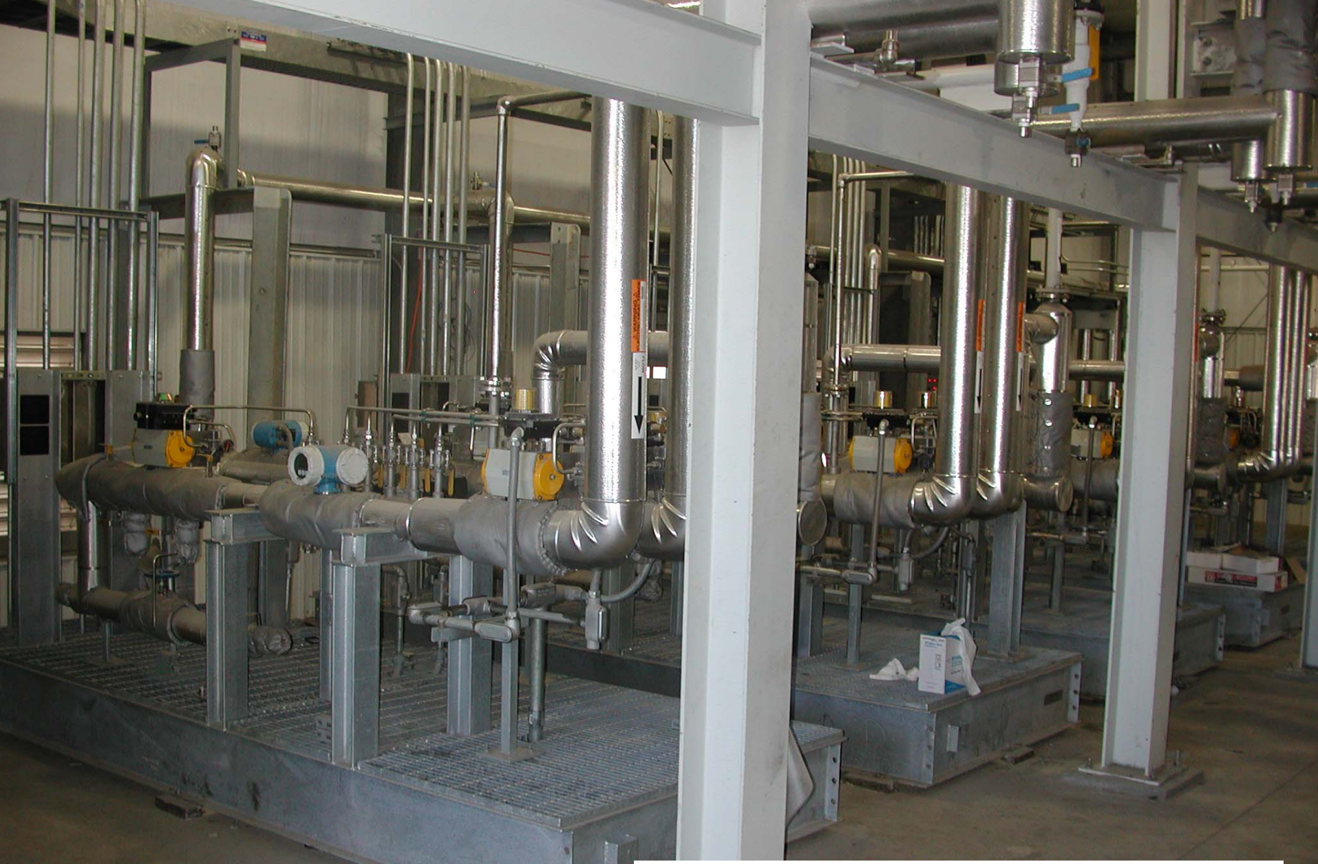
Injection Metering Skids
