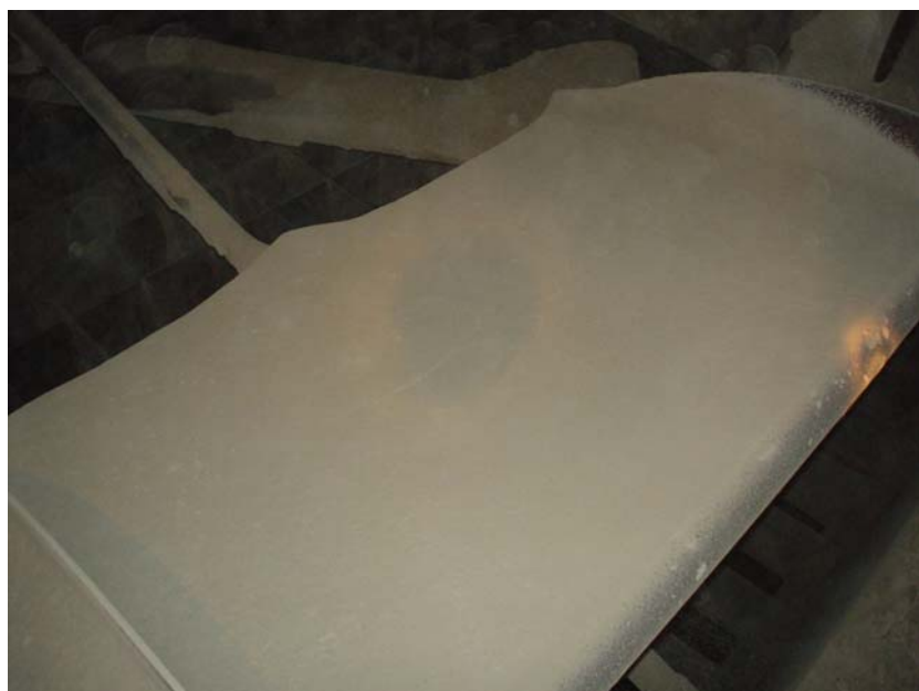
Ash Buildup on Vanes
